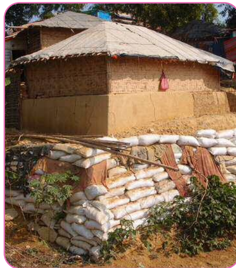
Fig. 14: Structure consolidation in refugee camps sometimes requires a lot of reinforcement. E. Cauderay, CRAterre, 2019.
